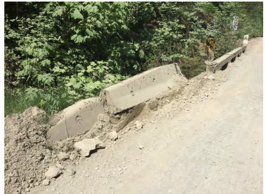
Upstream right approach misalignment
