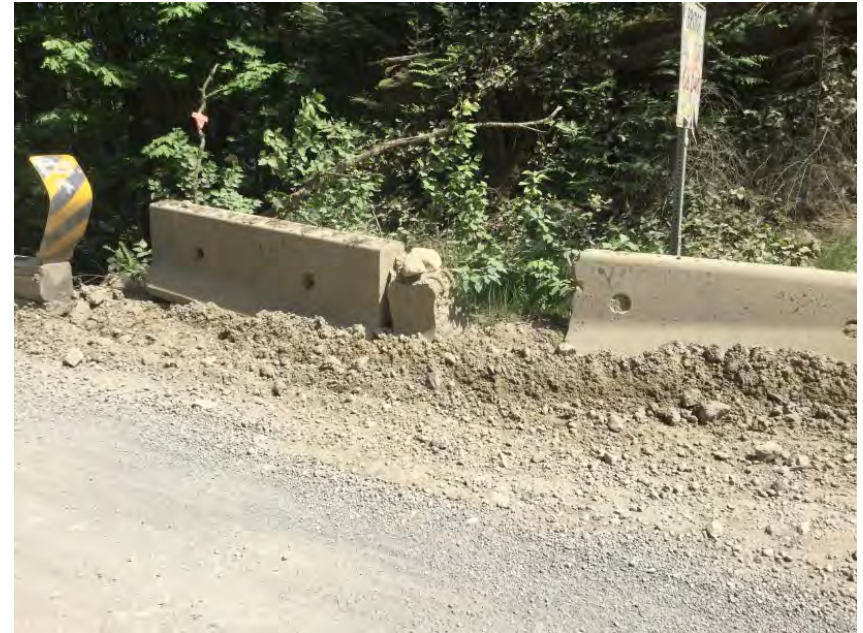
Downstream right approach barrier damage
